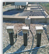
Elementary School, MO 3 Salcor 3G UV Units (Parallel Array) in Extended Aeration
