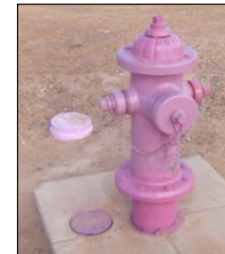
Reclaimed Water Fire Hydrant
