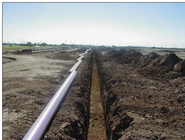
Reclaimed water pipeline, City of Chandler
