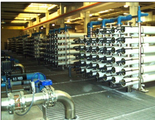
Advanced treatment of reclaimed water, Scottsdale Water Campus City of Scottsdale photo
