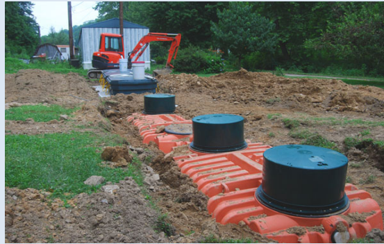
Septic tank, pump tank, and peat modules waiting Commission inspection
