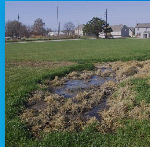
Failed System Renovation
